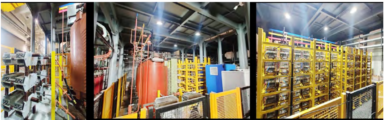
Figure B.11. The 55kV, 6MW MHVPS installed at ITER-India Power Supply Lab
