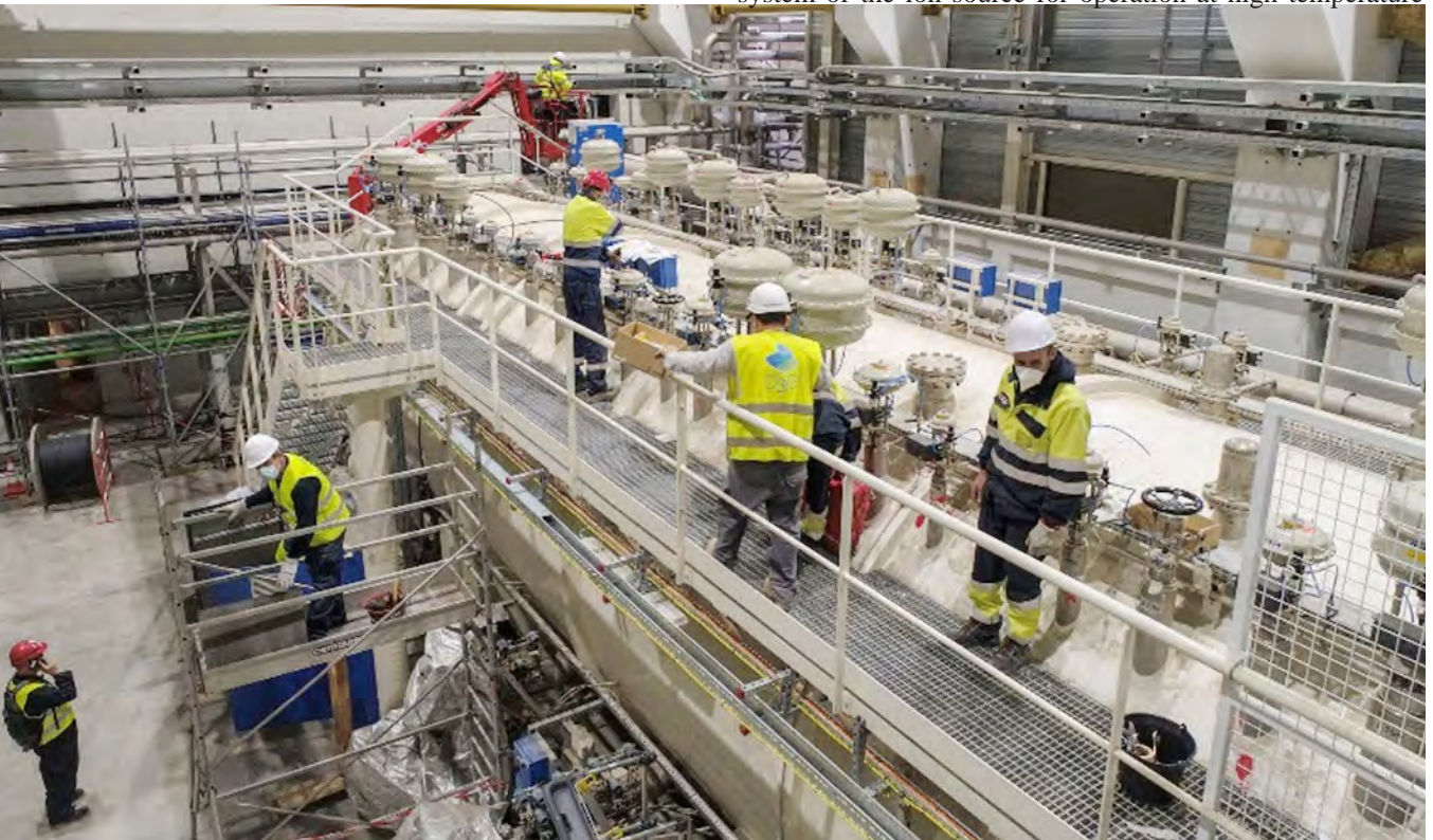
Figure B.6. Installation of 20 m long 3.5 m diameter 70 tonne cryoplant termination cold box (CTCB)
